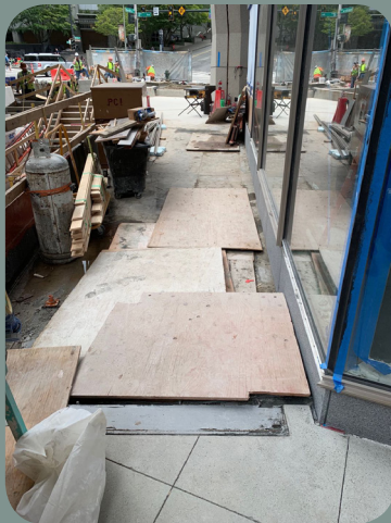
Uneven running slope
